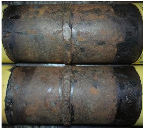
Figure 4: Girth Weld Area (External)
